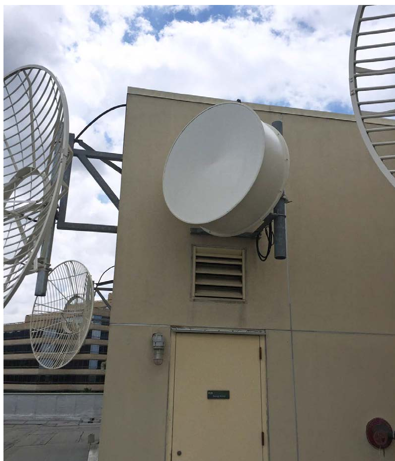
Part 101 now allows for use of 11 GHz, and high-speed IP radio links can be used to connect and extend AoIP networks such as those discussed here.
