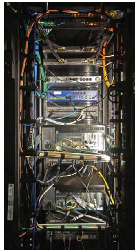
Built-in equipment rack lighting is a major plus.
